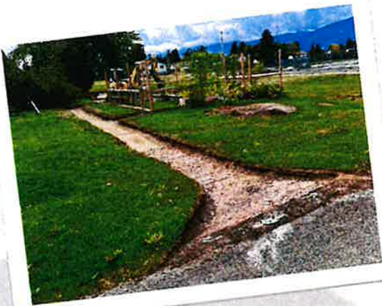
Progress is being made on the Nechako Elementary School Outdoor Learning and Cultural Space.
